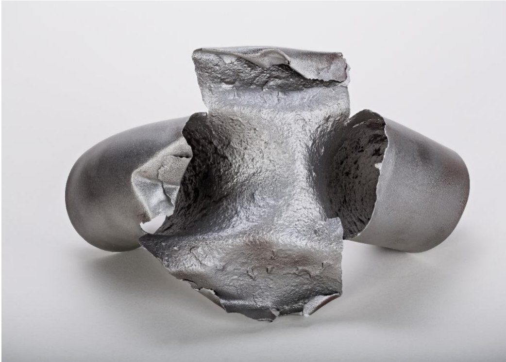
36 bar steam pipeline of a soot blowing system, the pipe bend burst as a consequence of internal erosion. Material: 15 Mo 3 (steel) © CEphoto, Uwe Aranas
