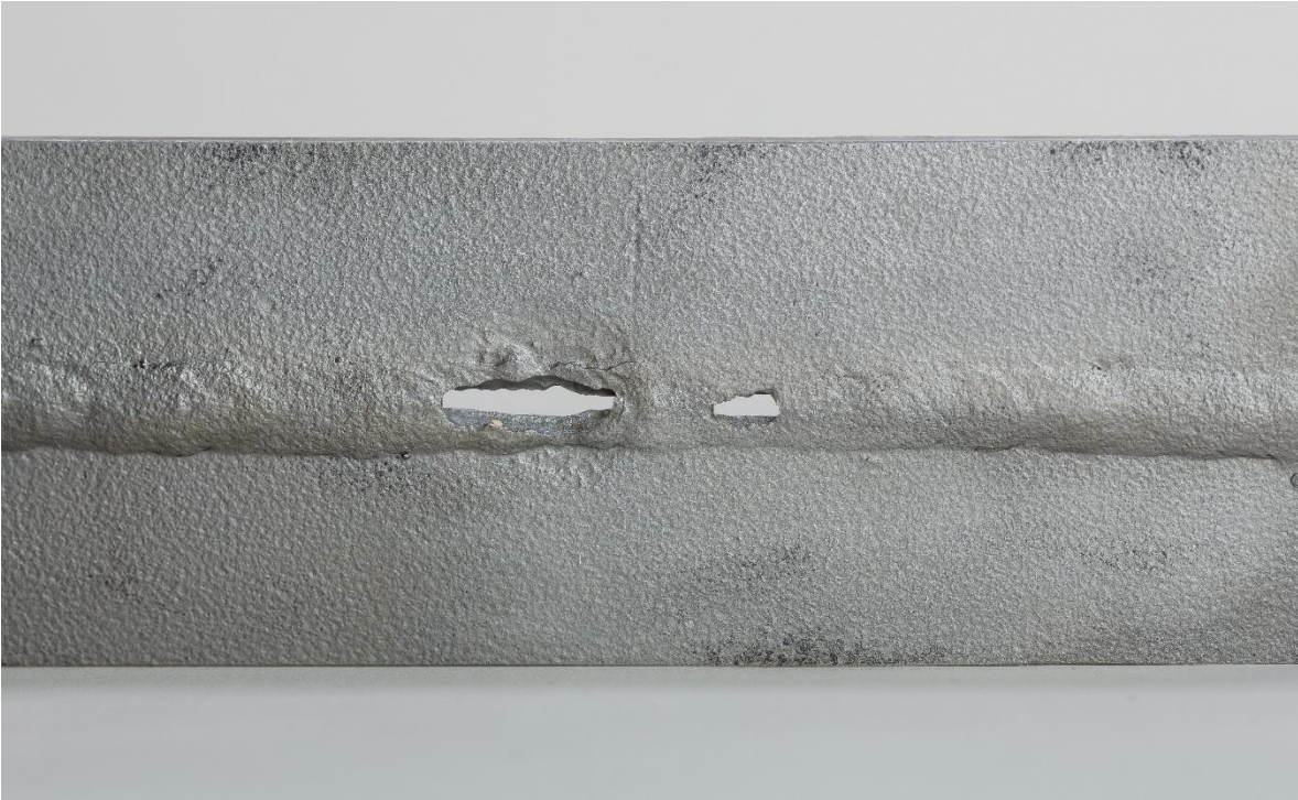
Damage mechanism: Acid corrosion in a flue gas duct as a result of condensation of flue gas. The acid accumulated behind the chamotte layer and caused the depicted corrosion. This photo: Atmosphere side of the duct © CEphoto, Uwe Aranas
