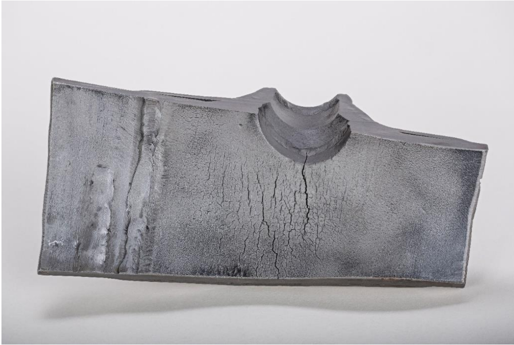
Damage mechanism: Stress corrosion cracking, caused by tension in an unsuitable welded reinforcement collar. No failure present © CEphoto, Uwe Aranas
