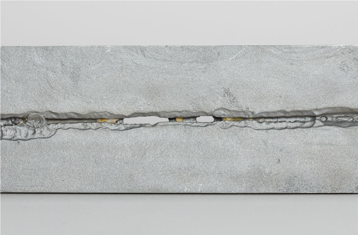
Damage mechanism: Acid corrosion in a flue gas duct as a result of condensation of flue gas. The acid accumulated behind the chamotte layer and caused the depicted corrosion. This photo: gas side of the duct © CEphoto, Uwe Aranas
