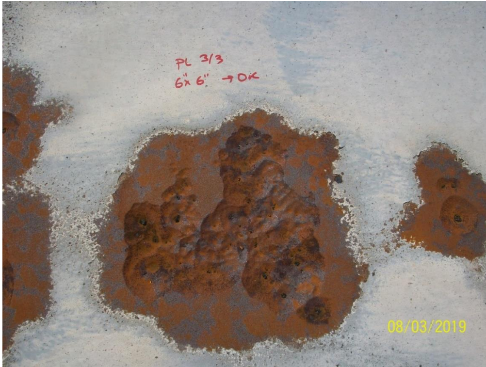
PICTURE 6. ATMOSPHERIC CORROSION IN THE EXTERIOR OF A TANK'S ROOF FOUND DURING AN INSPECTION. THE TANK WAS LOCATED IN A MARINE ENVIRONMENT, SO THERE WERE MANY OF THESE
