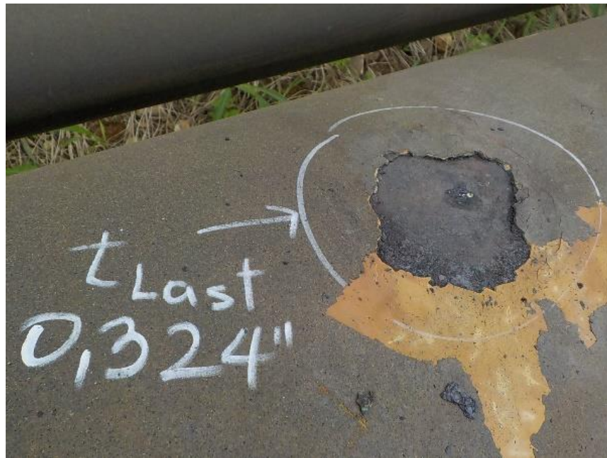
PICTURE 7. LOCALIZED COATING FAILURES IN A PIPE WILL PROMOTE LOCALIZED CORROSION
