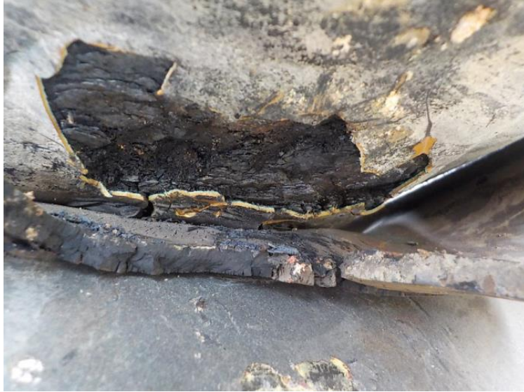
PICTURE 8. ATMOSPHERIC CORROSION IN THE LOCATION OF A SUPPORT IN A PIPE CLOSE. THE CORROSION RATE IS INCREASED BY A POND NEARBY
