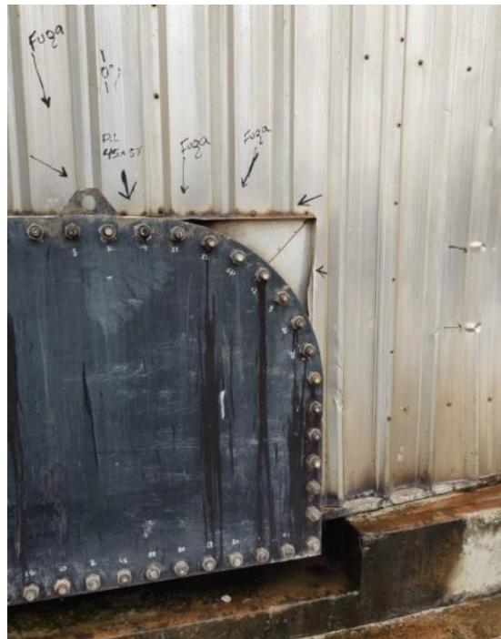
PICTURE 14. INSULATION POSSIBLY SHOWING MOISTURE PATHS ABOVE THE CLEANOUT DOOR
