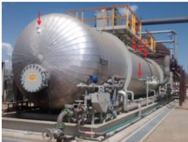
PICTURE 13. TREATER INSTALLED IN ONE OF THE AUTHOR'S PROJECTS, WITH DAMAGE TO THE INSULATION
