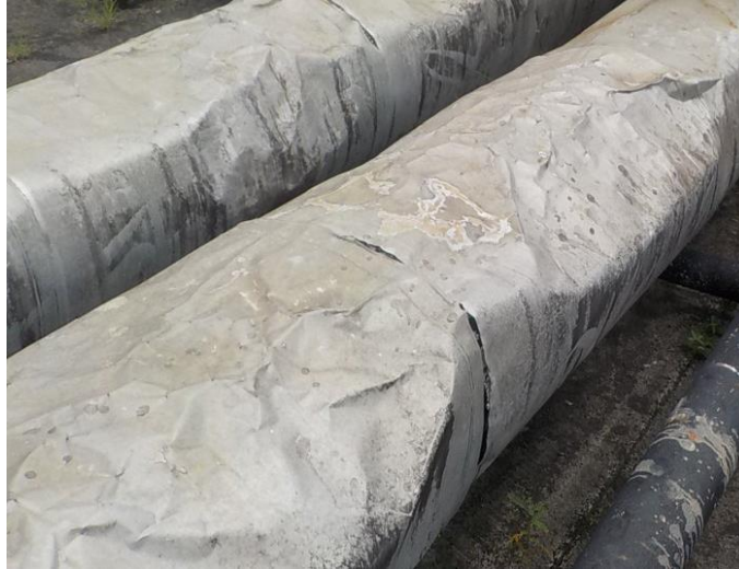
PICTURE 12. INSULATION DAMAGE IN PIPE SERVICING A TANK, BECAUSE OF PEOPLE STEPPING IN THE JACKETING
