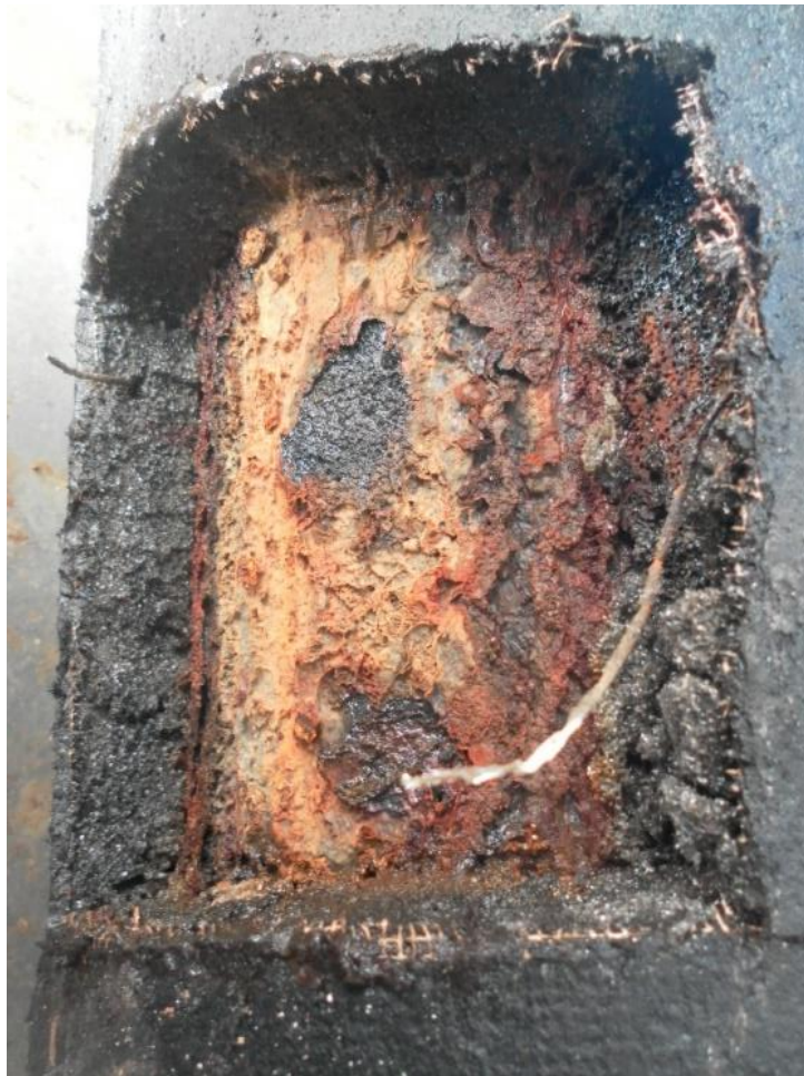
PICTURE 9. INSULATION WINDOWING IN A VERTICAL PIPE IN A PRESSURE VESSEL SHOWING CORROSION UNDER INSULATION IN THE LOWER PARTS OF THE LINE. MORE INSULATION SHOULD BE REMOVED.
