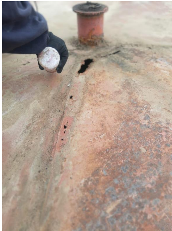
PICTURE 15. A HOLE IN A TANK'S ROOF, CAUSED BY CUI CLOSE TO THE SCAFFOLD CABLE SUPPORT
