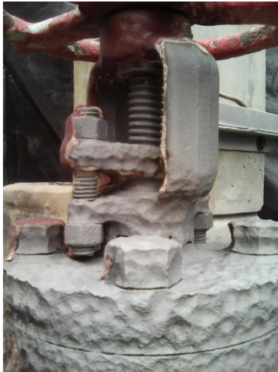
PICTURE 16. GATE VALVE SHOWING SEVERE CORROSION UNDER INSULATION IN A PETROCHEMICAL COMPLEX
