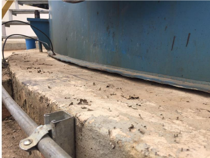
PICTURE 22. THE USE OF A BARRIER PREVENTING WATER INGRESS OR A VCI SYSTEM CAN HELP REDUCE SOIL CORROSION IN TANKS
