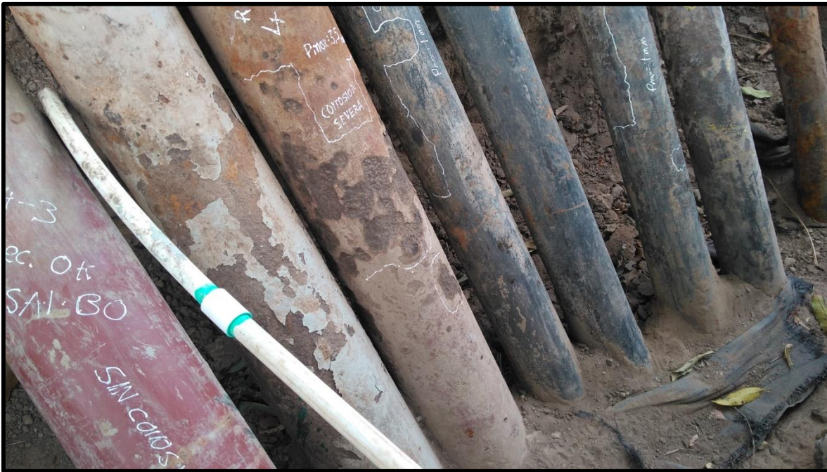
PICTURE 17. SOIL CORROSION IN THE INTERFACE OF BURIED PIPE INTERFACES
