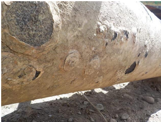
PICTURE 20. SEVERE SOIL CORROSION IN A BURIED PIPE IN A PROCESSING FACILITY
