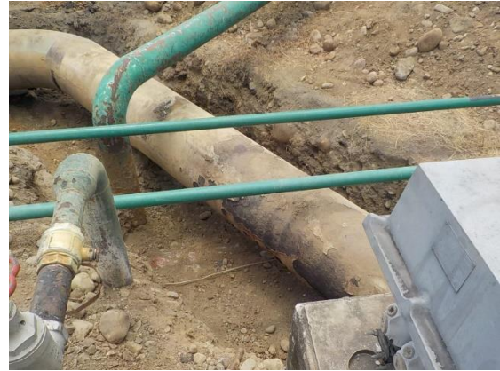
PICTURE 19. THIS PIPE LOOKS GOOD FROM A DISTANCE, BUT THERE IS SEVERE SOIL CORROSION UPON FURTHER EXAMINATION
