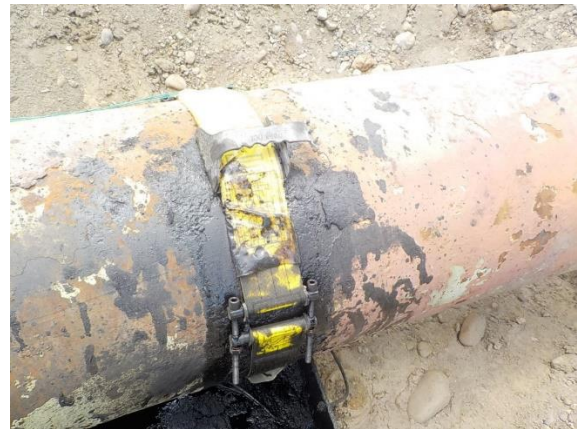
PICTURE 21 TEMPORARY FIX IN A LEAK RESULTING FROM SOIL CORROSION
