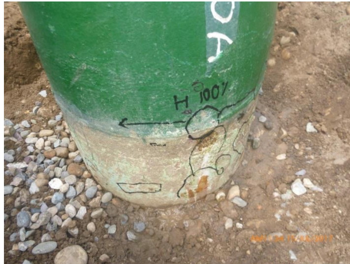
PICTURE 23. INTERFACES SHOULD BE EXCAVATED 12 IN. (305 MM) BELOW THE SURFACE TO EXPOSE THE MOST CORROSION-PRONE AREA
