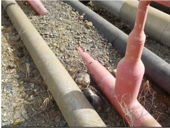
PICTURE 18 SOIL THAT HAS ACCUMULATED OVER A PIPE
