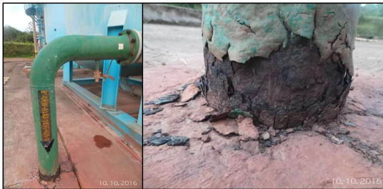
PICTURE 24. A INTERPHASE CORRODING IN A POTABLE WATER TREATMENT SYSTEM
