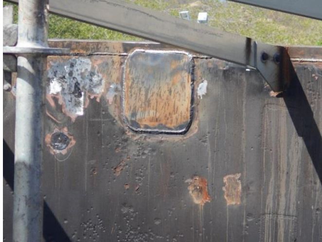
Picture 2. LAPPED PATCH ON THE SHELL, NEXT TO THE ROOF. OTHER CORRODED AREAS CLOSE TO THIS PATCH WHERE FILLED BY WELDING
