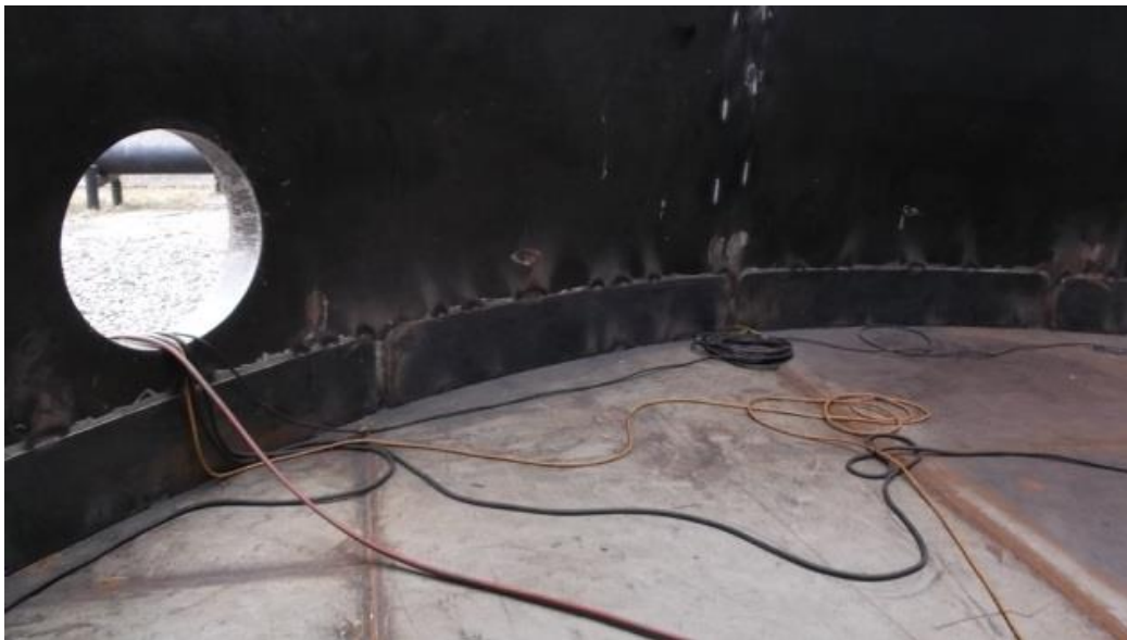
PICTURE 2. TOMBSTONE LIKE LAPPED PATCH PLATES WELDED IN THE INSIDE OF A TANK SHELL. THE PATCHES ARE BIGGER THAN ALLOWED BY API 653. IT WORKS, ANYWAY.
