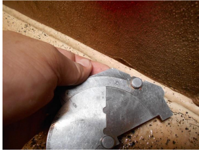
PICTURE 1. LACK OF MATERIAL IN THE SHELL ADJACENT TO THE SHELL-TO-BOTTOM WELD. CASE 4 (ANY OTHER INTEREST AREA)
